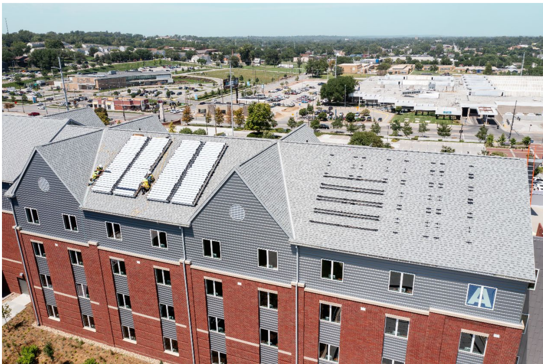
Graves Hall - VIRTU HOTHD Installation
